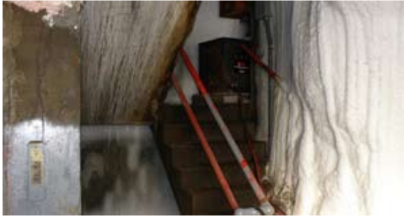
Ice Buildup Blocking Stairway
